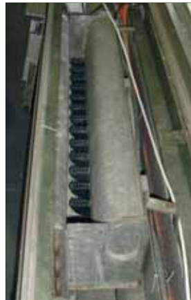
Induction units in the offices
